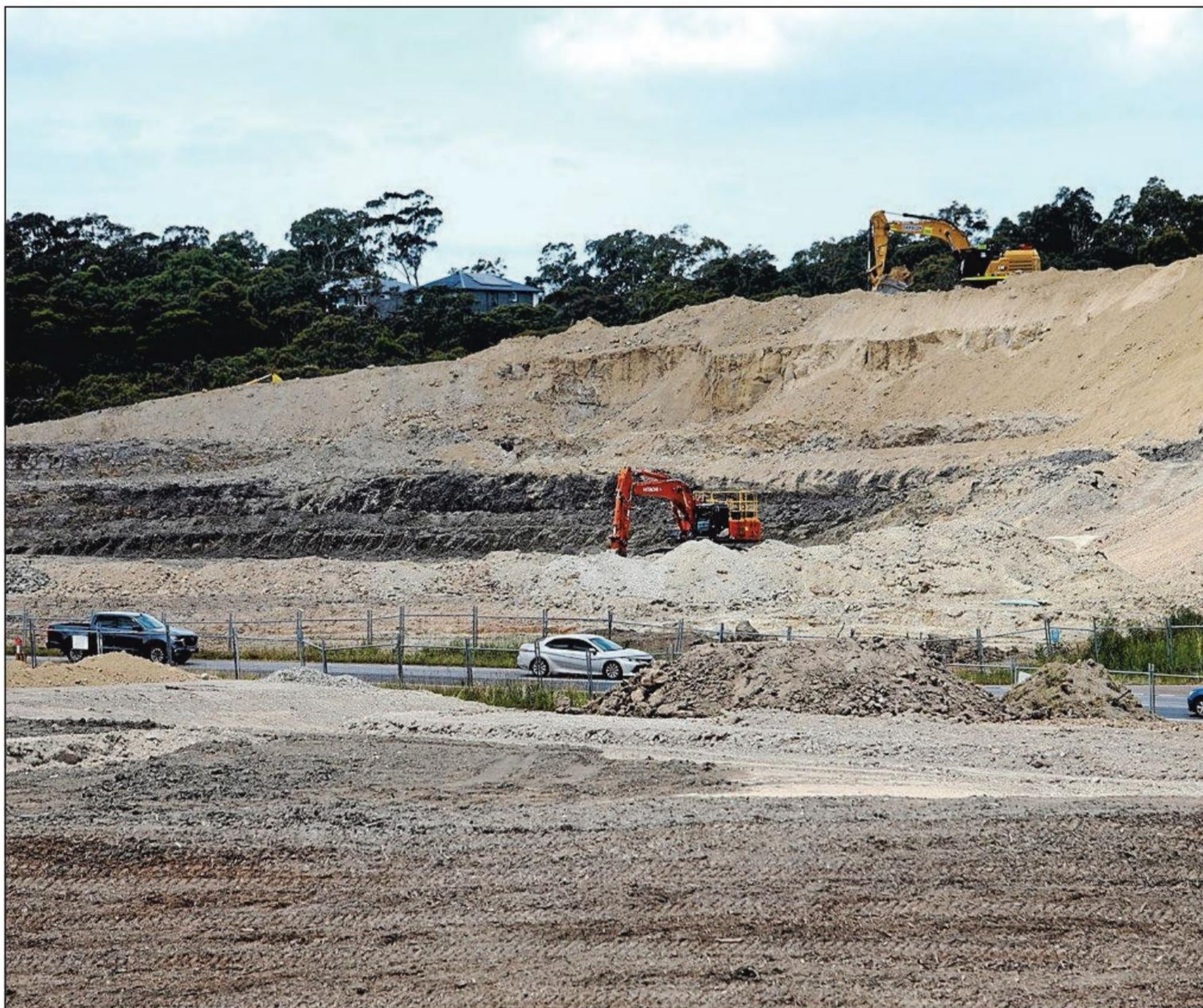
Land clearing currently underway on the eastern side of Minmi, which will form part of the housing estate. Picture by Peter Lorimer
